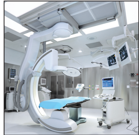
Hybrid Operating Room
